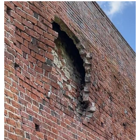
Figure 23 Damage to the protective wall of the Castle of the Dukes of Mazovia in Czersk. (photo by B. Szostak)
