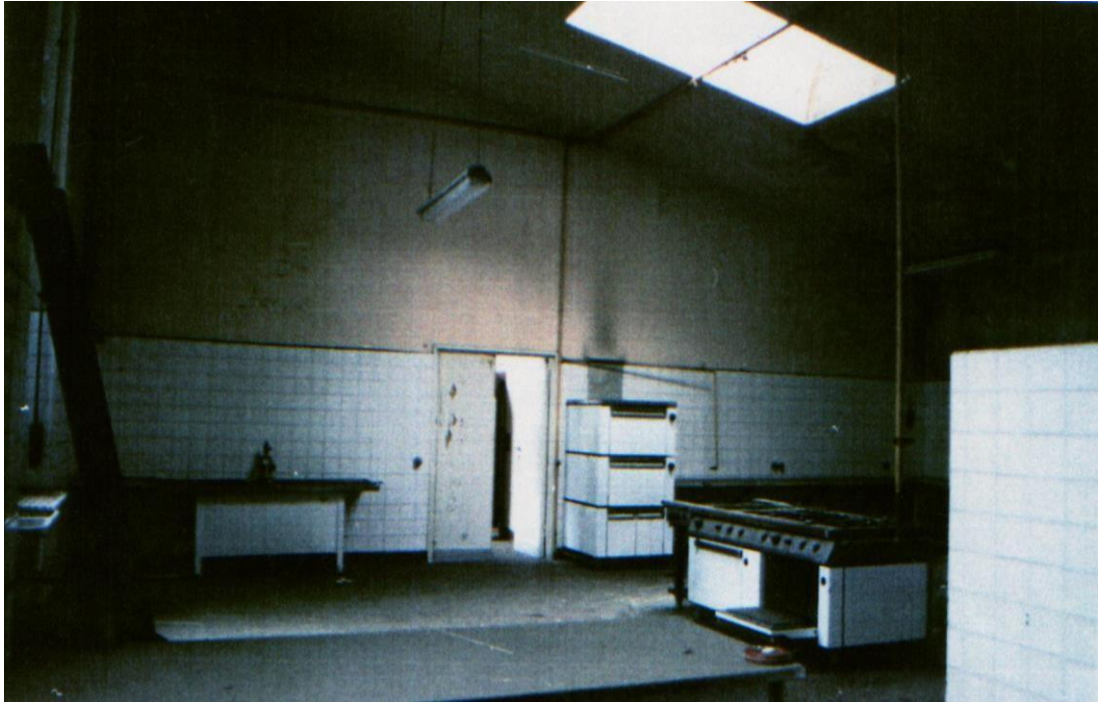
Figure 12 Colonia Elioterapica in 1988: view of the abandoned kitchen.
