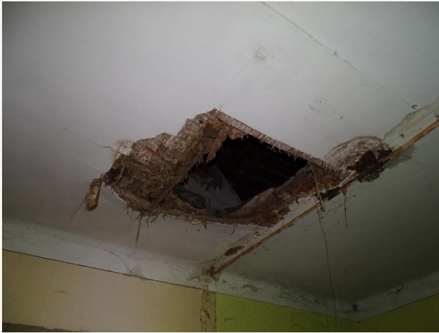
Figure 10 No possibility to make inventory of attic because of damaged ceiling – the historic forester's lodge in Łopiennik Dolny, Poland.
