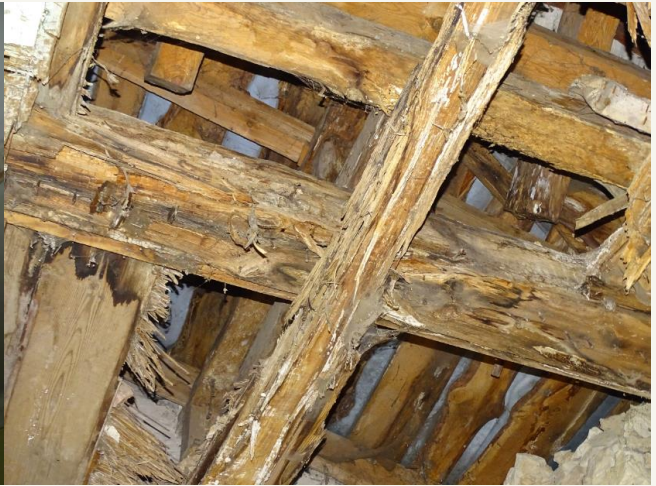
Figure 11 Lack of access to the roof truss due to its complex layout – the historic forester's lodge in Łopiennik Dolny, Poland.
