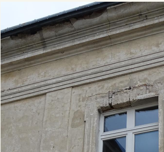
Figure 6 Visible protection of the cornice fragments with a mesh – the Zamoyski Palace in Zamość, Poland.
