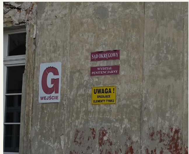
Figure 7 Marking – "Attention! Falling plaster fragments". – the Zamoyski Palace in Zamość, Poland.
