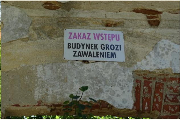
Figure 9 Marking – "No trespassing – building in danger of collapse" – the Szreńsk Castle, Poland.
